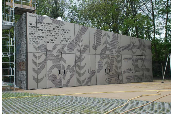
The access doors to the kiosk subtly integrated into the art installation. Credit: Thames Tideway
