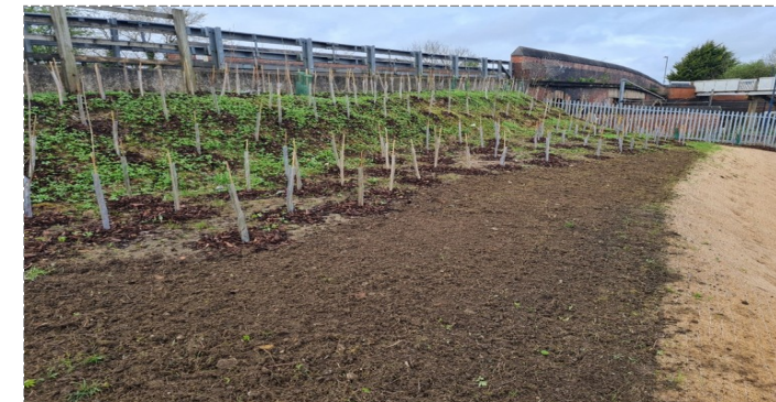
Area seeded with wildflower mix and use of biodegradable coir matting on embankment (March 2024).
