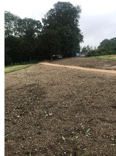
Photo Description: S&T(UK) prepared soils post drainage works to allow them to carry out planting.
